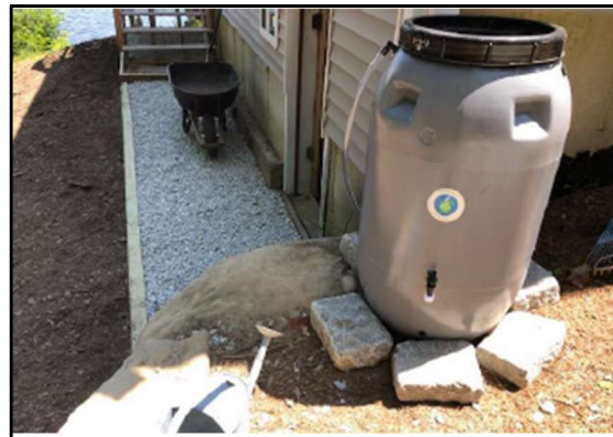
Rain barrel and dripline trench installed to capture and infiltrate roof runoff
