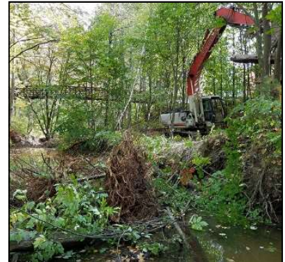
Contractors install rootwads and woody debris in the stream to create habitat and restore floodplain connectivity.
