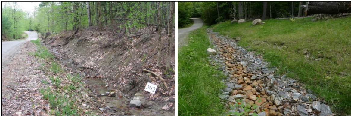
Cochrane Drive - Extensive bank and ditch erosion (left) was addressed by reshaping the steep bank; seeding and mulching the new slope; and arming the ditch with riprap (right).
