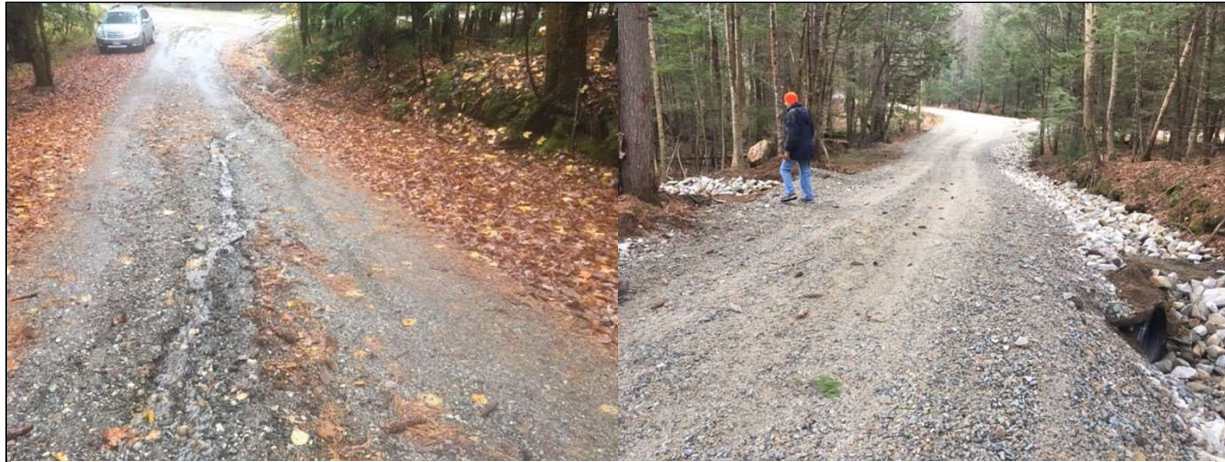
Prior to the project, Beaver Way experienced chronic erosion with direct flow into the lake (left). Several BMPs were installed including two culverts, riprap-lined ditches, two turnouts and a rubber razor (right). Pollutant loading was reduced by an estimated 17 tons of sediment and 14 pounds of phosphorus.
