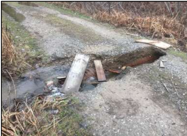
Before: Failed culvert; driveway washed out
