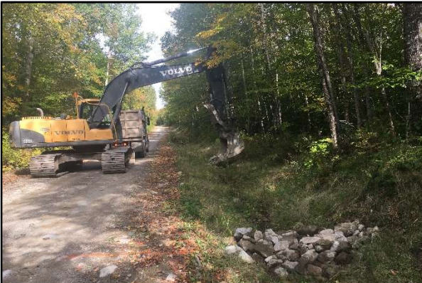
Birch Lane ditches armored with stone and seed/mulch and check dams installed.
