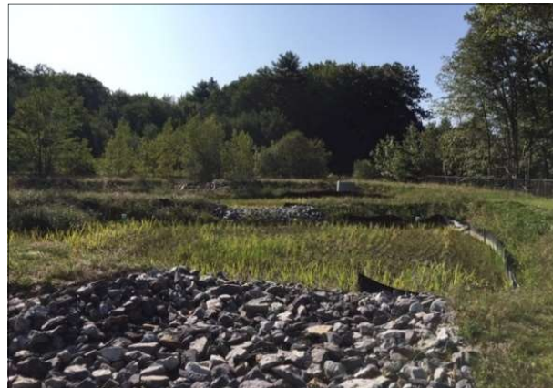
Gravel wetland installed as part of the Private Property Matching Grants task.
