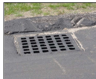
Sealant applied to parking lot draining to Thatcher Brook in Biddeford.
