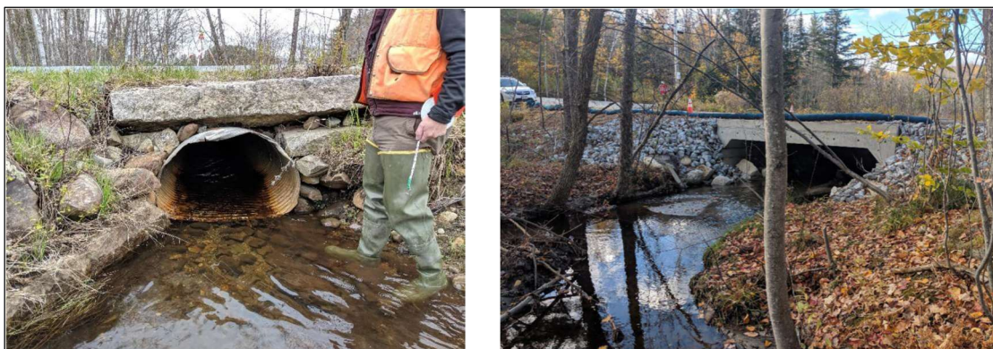
The Town of Wilton received an $80,000 culvert grant to replace the undersized and unstable culvert on Pond Road (above left) with a 17.5-foot wide open-bottom concrete box structure (above right). The project provided fish habitat, water quality, and climate resiliency benefits.
