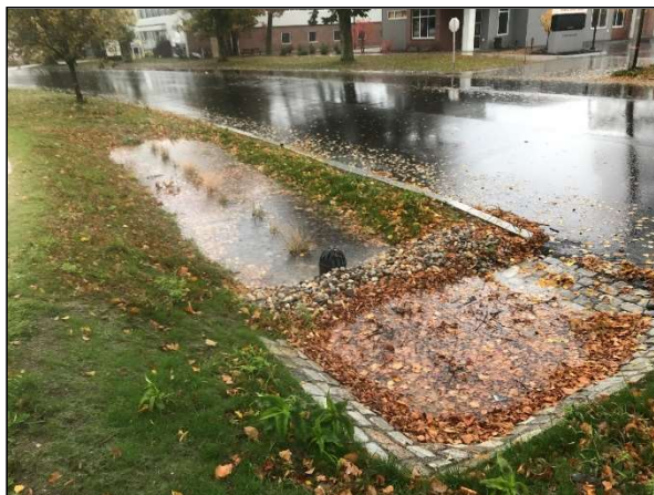
One of six under-drained soil filters installed to treat stormwater in the City of Portland.
